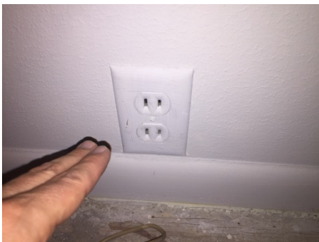
Attic: painted outlet
