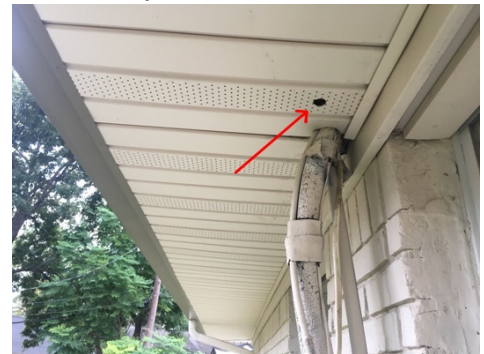
Left: hole in soffit
