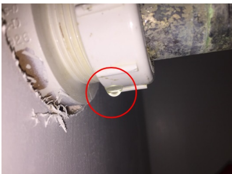
Bathroom 2: leak at drain
