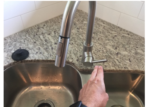
Kitchen: no cold water at faucet
