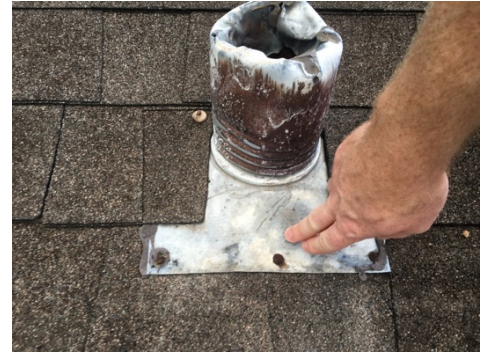
Exposed nail heads
