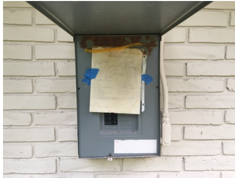
Rear: service panel
