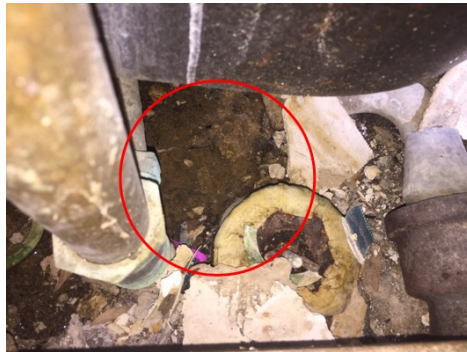
Bathroom 1: water under tub near drain
