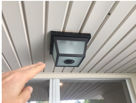
Front porch: inoperable light fixture
