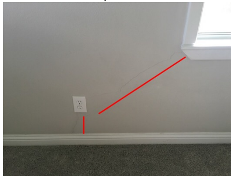
Bedroom 1: diagonal crack
