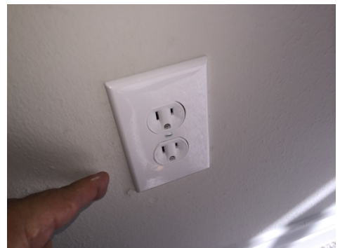
Bedroom 2: Loose outlet
