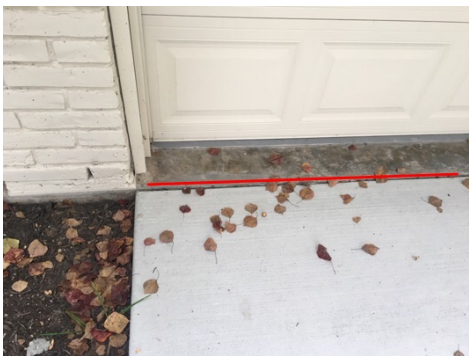
Driveway/walk to foundation: Monitor area for insect activity
