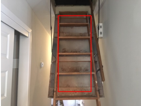
Pull-down stairs/scuttle panel lacked insulation
