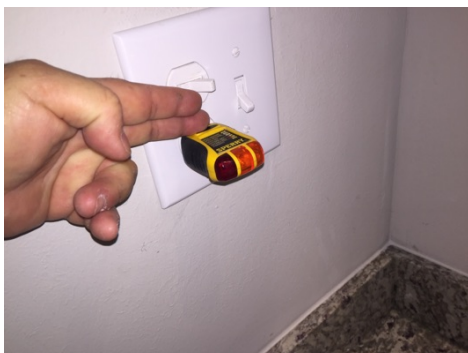
Bathroom 1: Outlet not GFCI protected to the left of the lavatory
