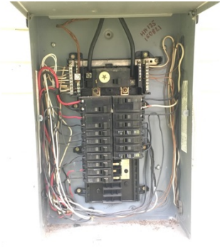
Rear: service panel
