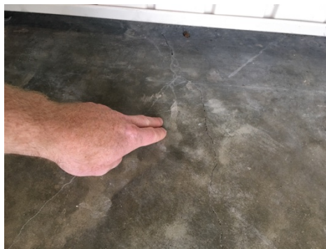
Entry: hairline crack
