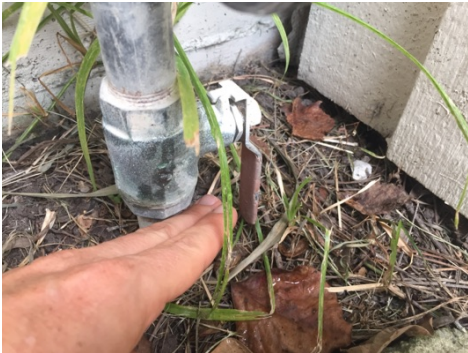
Right: Main Water Shutoff valve
