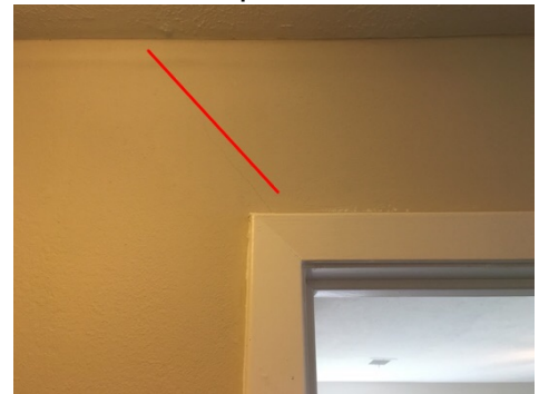
Hall: Diagonal crack
