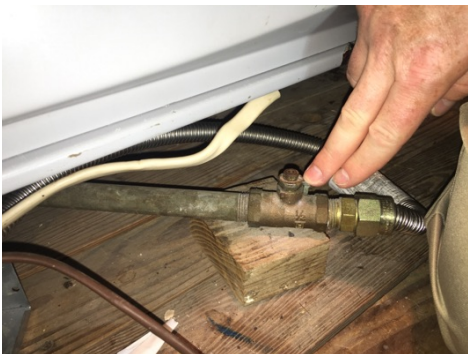
Shutoff valve damaged REI 7-5 (05/4/2015)
