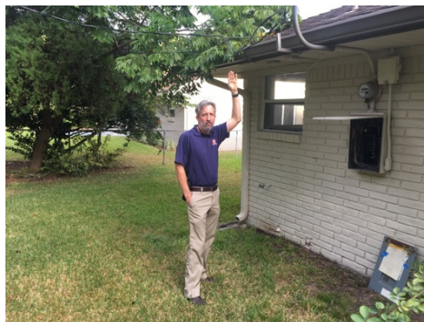
Service too low
