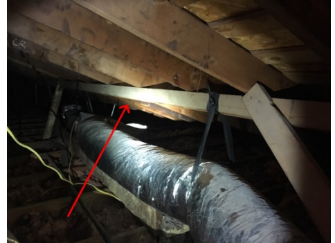
Undersized purlins - insufficiently supported
