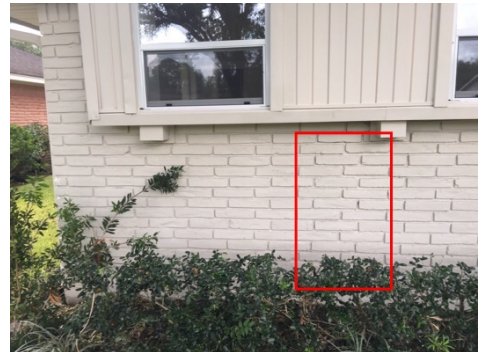
Front: Step crack
