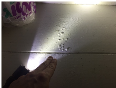
Bathroom 1: water on cabinet floor from leak at drain
