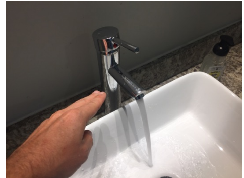
Bathroom 1: loose faucet
