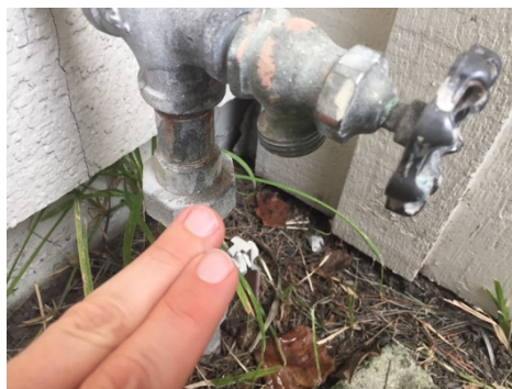
Around house: Back flow preventer recommended
