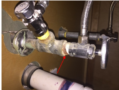
Kitchen and bathrooms: dissimilar metals in contact
