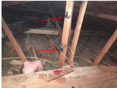
Photo eye sensor in the attic were more than 6" off ground
