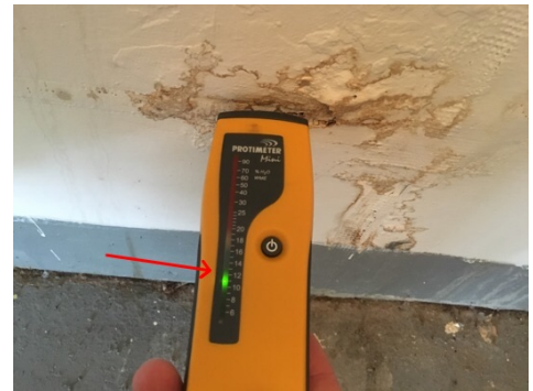
Garage laundry room: Moisture stain and damage dry at time of inspection
