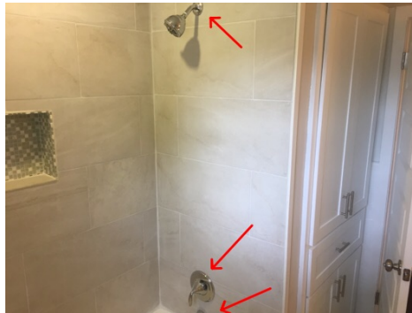
Bathroom 1: missing caulk at wall protrusions
