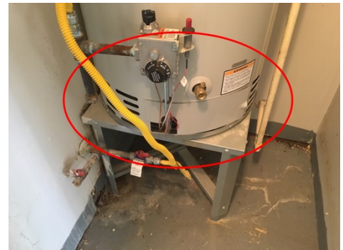
Missing safety pan
