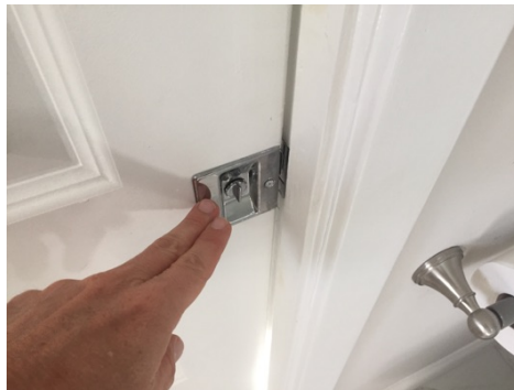
Bathroom 2: would not latch
