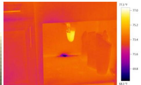
Bathroom 2: water on cabinet floor from leak at drain
