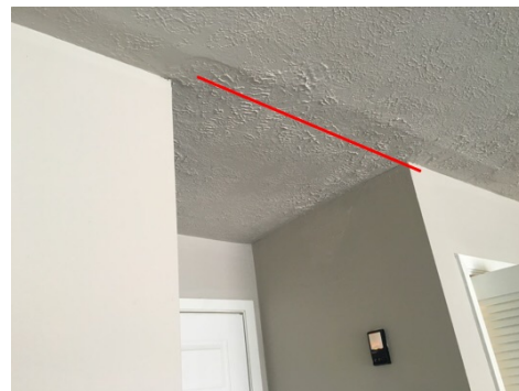
Garage: Hairline crack
