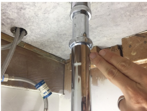
Bathroom 1: leak at drain stem
