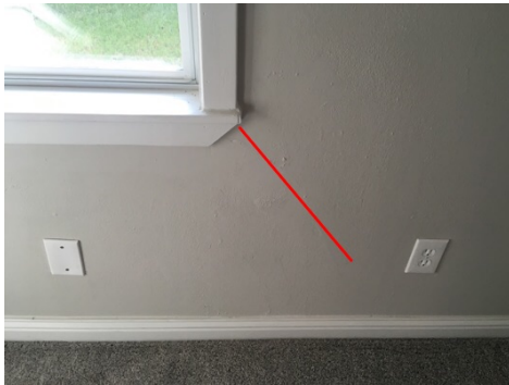
Bedroom 3: Diagonal crack
