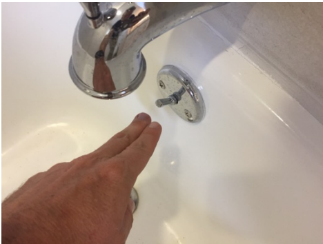
Bathroom 1: drain stop at tub would not retain water
