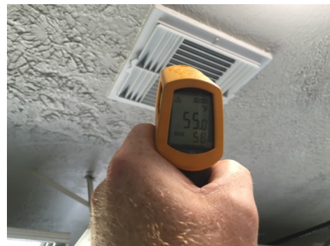
Garage: active vent
