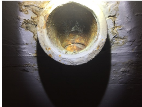
Garage: cast iron drain
