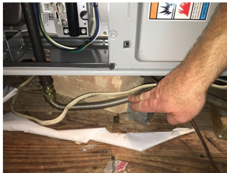
Missing drip leg
