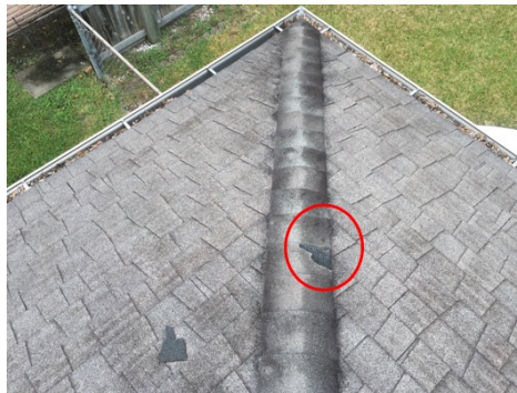
Rear left: torn shingle
