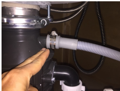
Drain Knock out at garbage disposal still in place
