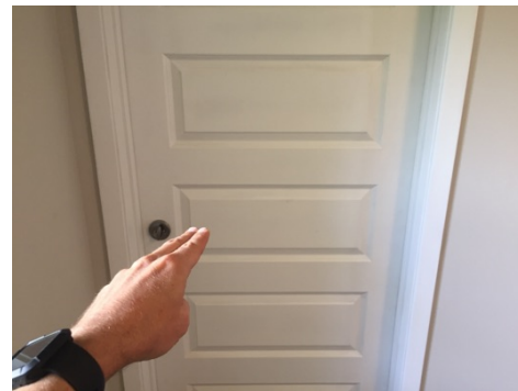
Garage man door: not fire rated
