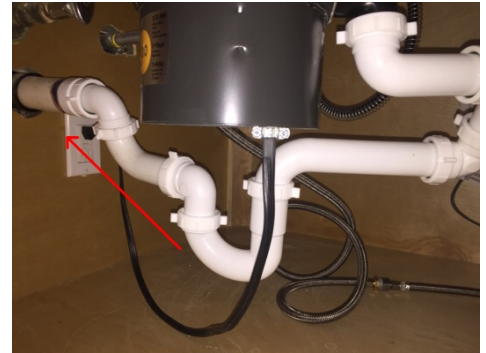
Kitchen: improperly sloped drain line
