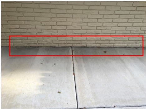
Rear: blocked weep holes
