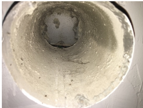
Dryer vent clear
