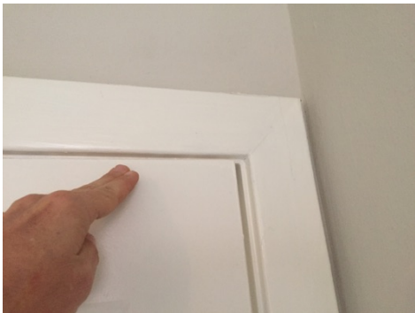
Bedroom 3: door rubbed on frame and out of square
