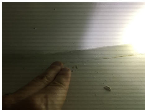
Bathroom 2: water on cabinet floor from leak at drain
