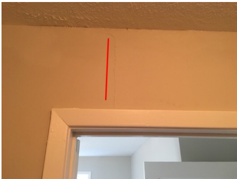
Bedroom 1: Hairline crack
