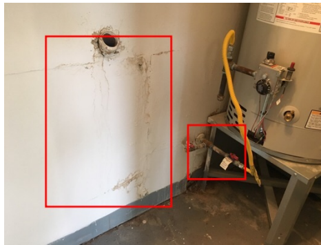
Garage laundry room: Moisture stain and damage dry at time of inspection
