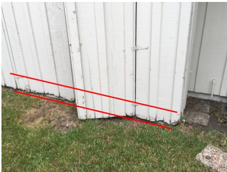
Right: wood decay
