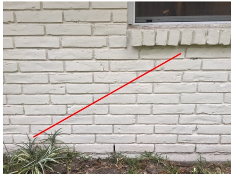
Rear: step crack
