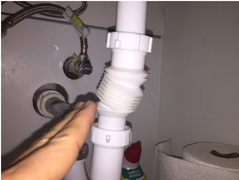
Bathroom 2: corrugated drain line
