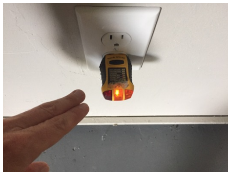
Garage: open ground at multiple outlets
