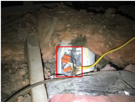
Attic: open junction box
