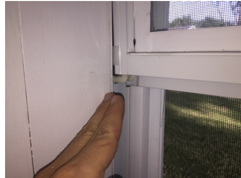
Bedroom 1: loose hardware at left front window
