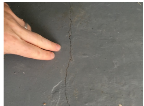
Garage: Hairline crack
